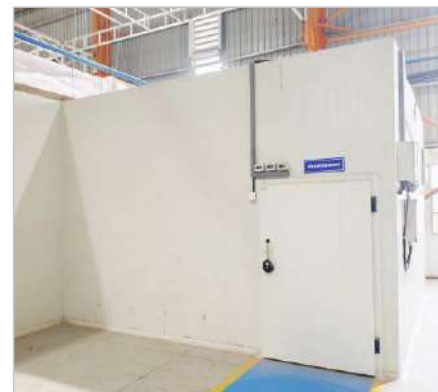
Cold Storage (-18°C)
